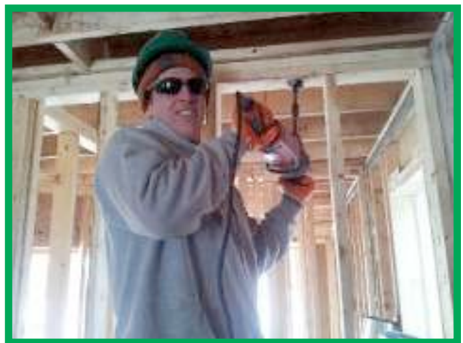
Top: Students in the Specialist High Skills Major Program helped build a home through Niagara Catholic's Raise Me Up Initiative.
